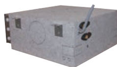
Metal parts insulated to avoid condensation
